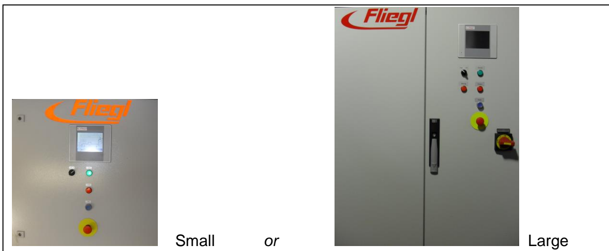
Figure 2: Safety and monitoring devices
